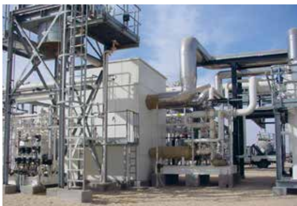
Outside installation: adapted to climatic conditions
